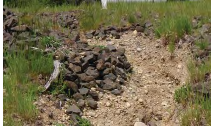
Erosion damages this dissipator.
