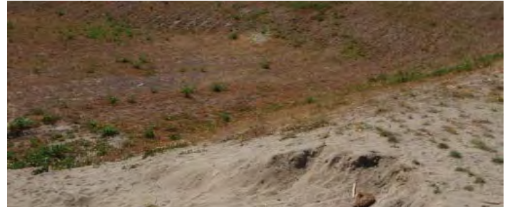
This berm is experiencing erosion.
