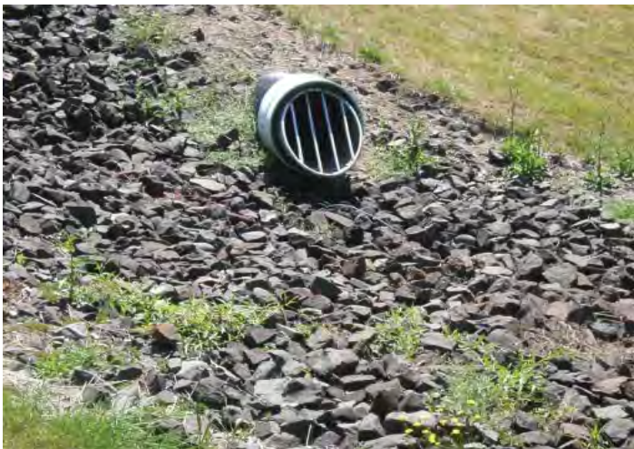
A well-maintained inlet pipe
