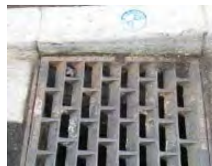
Functioning catch basin
