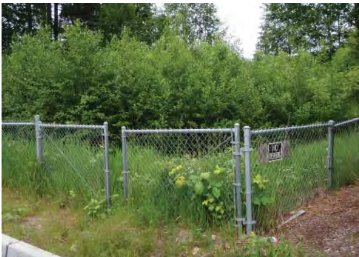
Alders and blackberry bushes have taken over this dry pond, hindering the infiltration of water.
