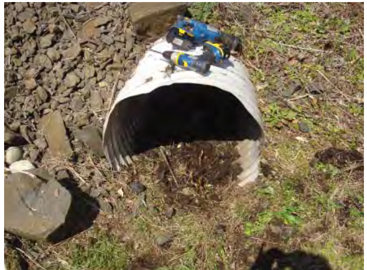
This inlet lacks a trash rack and is loaded with sediment.
