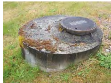
A typical metering device
