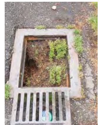
Catch basin clogged with sediment and debris
